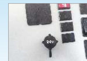
Mobile charging point
