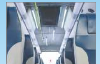
Eye-friendly LED roof lighting
