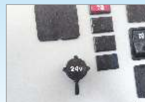
Mobile charging point
